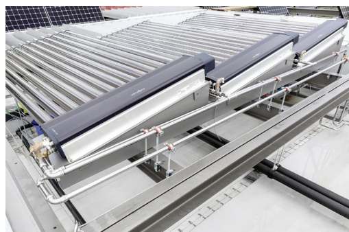
Img. 82 + 83 Solar thermal collectors
