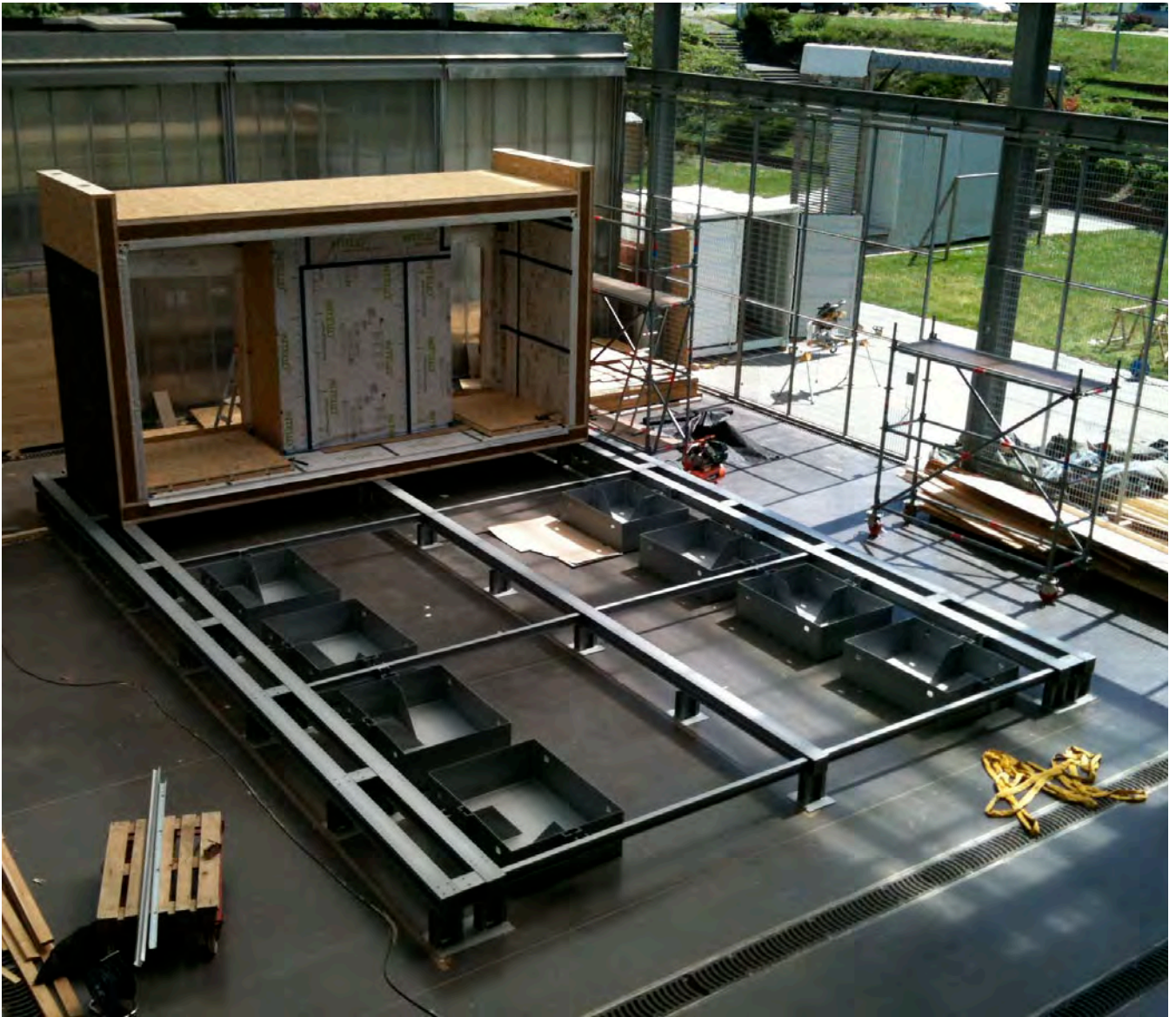
View of Armadillo Box® footing system under construction (mid April 2010) Lateral load stabilizing ballast sand boxes can be seen in place
